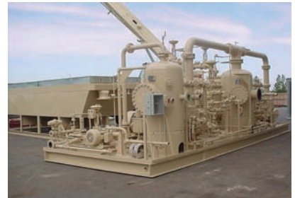
2004 South America installation. Dual rotary screw – 1.8 MMSCFD @ 250 psi (x2)
